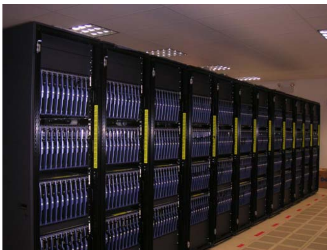
Maui High Performance Computing Center 1280 servers, Mellanox InfiniBand interconnect, 42.3TFlops
